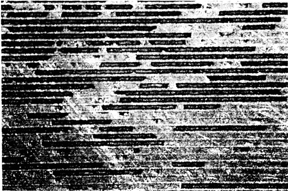
SURFACE DAMAGE CAUSED BY REMOVAL OF OVERLAY
