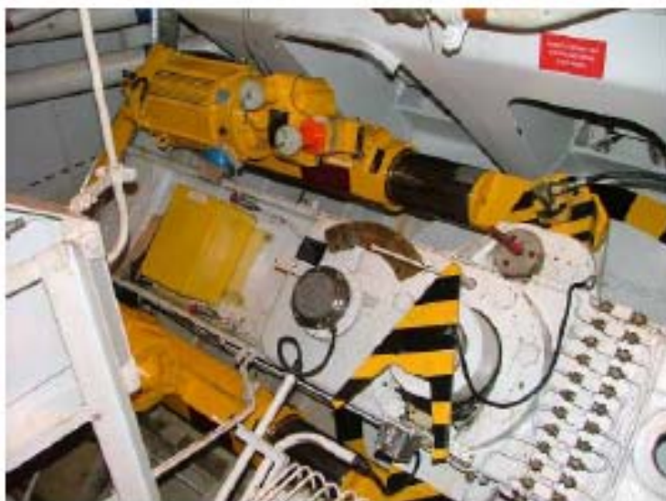
FIG.1 – ELAHCS GENERAL SURFACE VARIANT DRIVING A TYPE 23 FRIGATE'S PORT STABILISER
