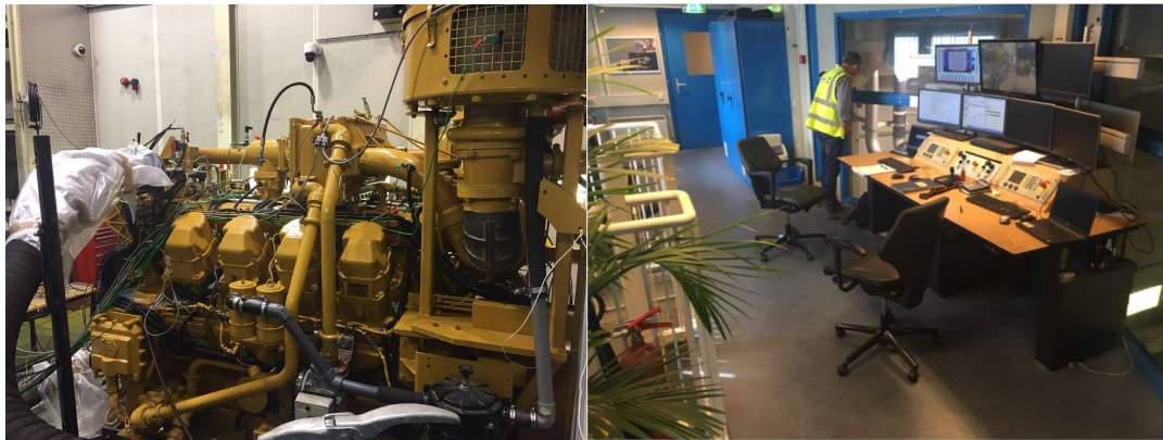
(a) (b) Figure 2: The converted CAT G3508A SI engine (a) and control room (b).
