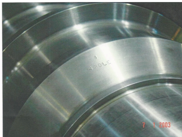
Figure 31: Mark on the generator shaft indicating a N -pole position.
