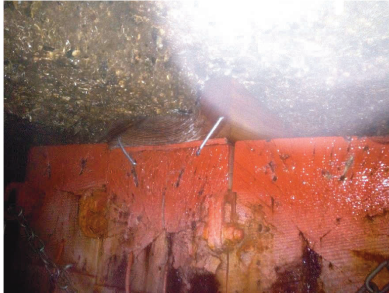
Figure 5: Wood in “crush” region
