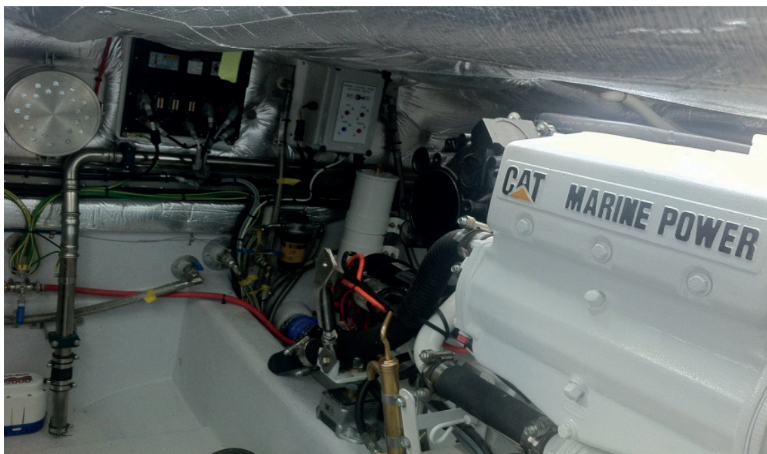
Figure 6 – Aerosol generator fitted in a small craft machinery space (top left of photograph)
