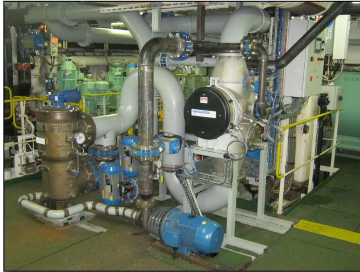
Figure 3. Typical BWMS Installation. Photo by Hyde Marine
