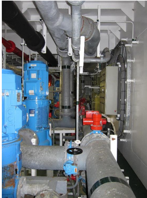
Figure 3. Forward Ballast Pump Space
