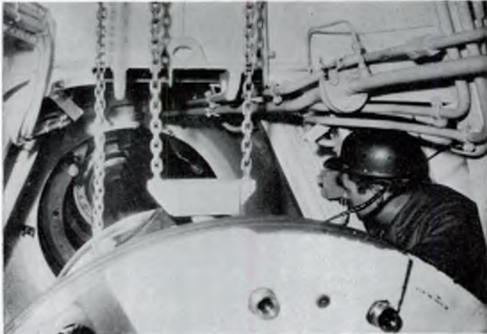
FIG. 11—Bearing withdrawn: inspector is in recess examining surface of outboard bush and shaft (If necessary the bush can be withdrawn along shaft to permit inspection of flange fillet).
