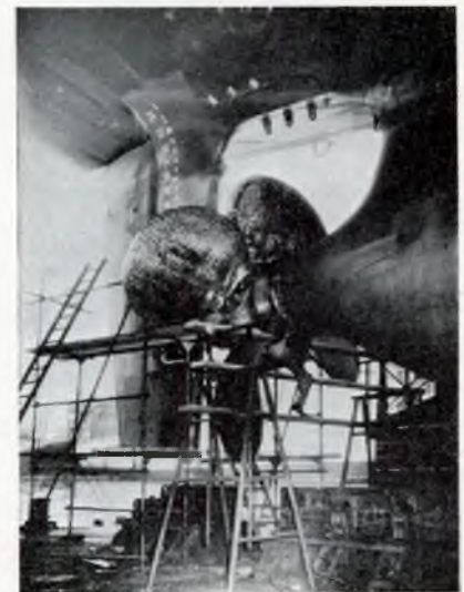
FIG. 14—Fitting propeller: hatch through which individual blades may be lifted to deck can be seen
