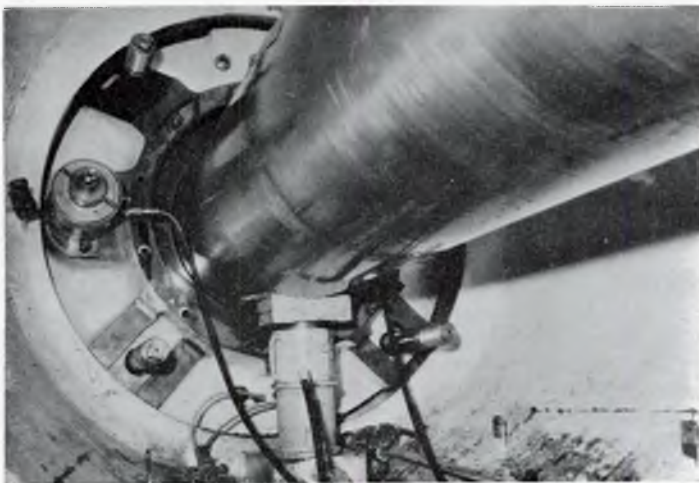
FIG. 13—Replacement of bearing—jack raising shaft from aft support to centralize and slide bearing home
