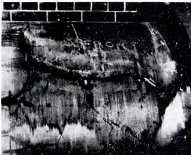
FIG. 3—Thermal cracking of a liner
