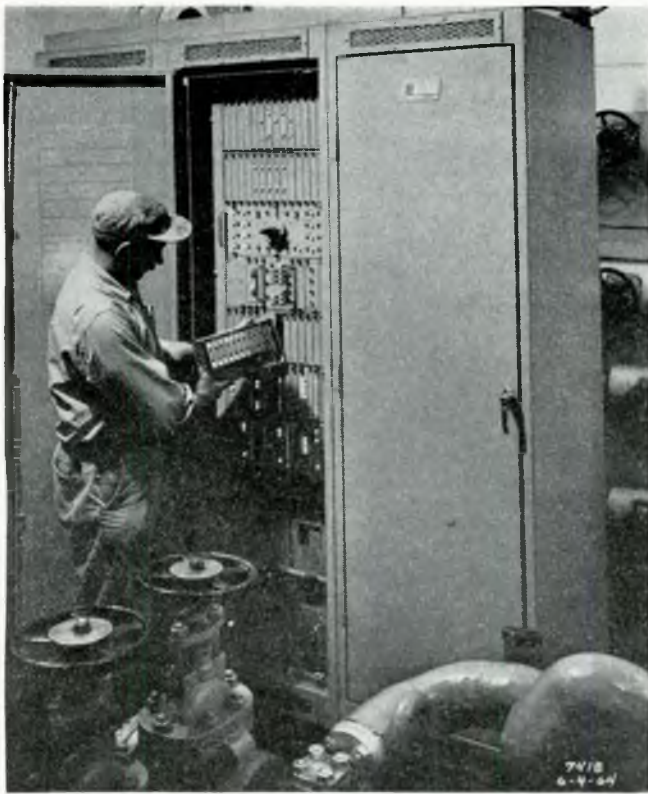
FIG. 17—Data processing cubicle
