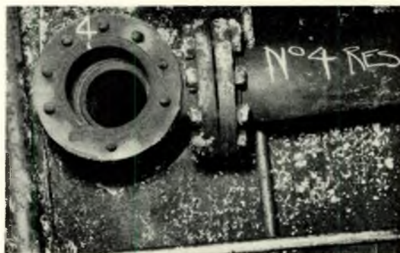
FIG. 2a—Port main engine room main air receiver—Main stop valve and pipeline
