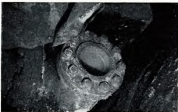
FIG. 2e—Port generator room main air receiver— Damaged first section of main air line, scorched air receiver and pipeline flange
