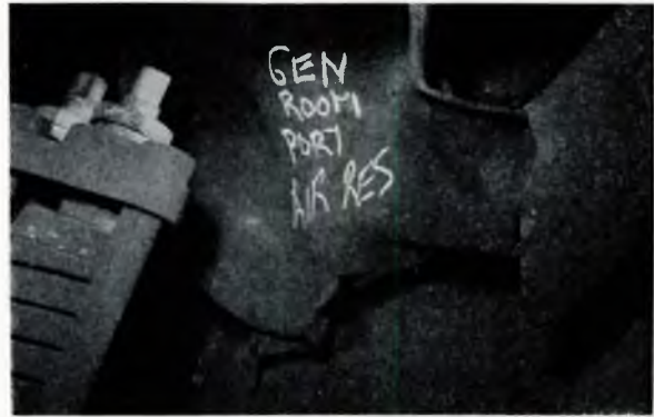
FIG. 2f—Port generator room main air receiver— —Damaged first section of main air pipeline from main stop valve
