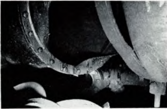
FIG. 2c—Starboard main engine room—Damaged scavenge air blower outlet trunking and starboard main air line “T branch”
