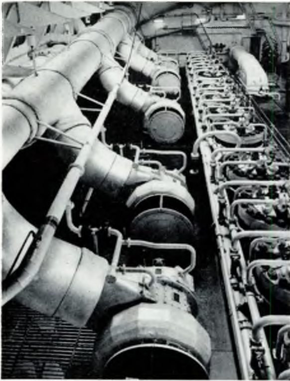
FIG. 5—Fiat engine type 9012S—View of cylinder heads photographed in the engine room of m.t. Carlo Cameli
