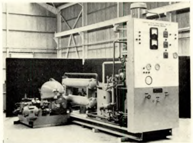
FIG. 3—General view of water washing plant
