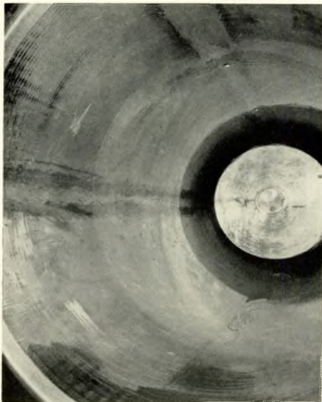
FIG. 23—Looking into the main tailshaft bush from the after end. The upper and port side oil grooves can be discerned by the light bearing and hand tool marks (done prior to fitting). A puddle of lubricating oil is visible below the tailshaft end
