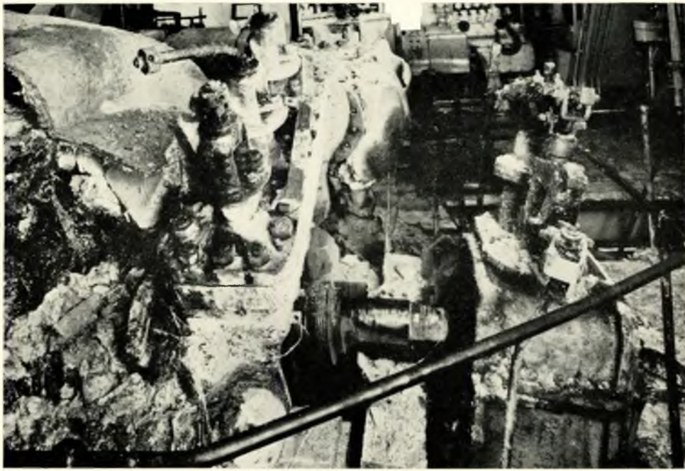
FIG. 4— Main turbo-alternator failure
