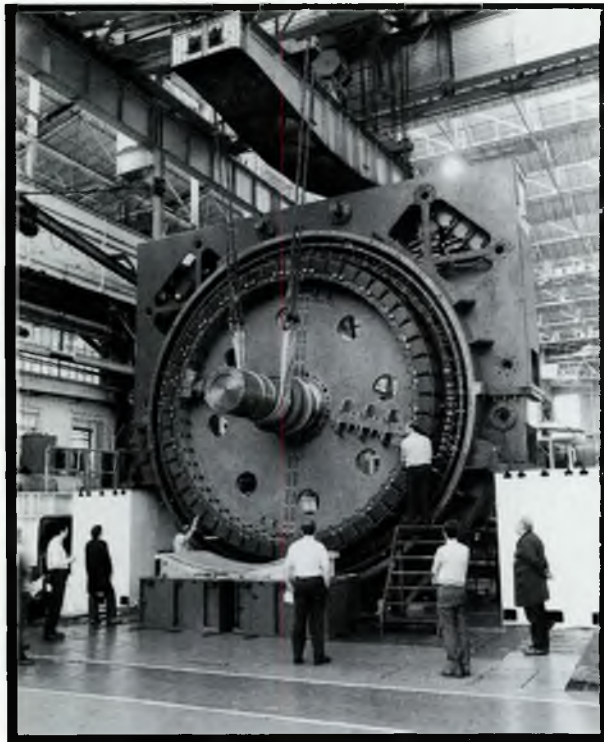
Fig. 22. QE2 propulsion motor
