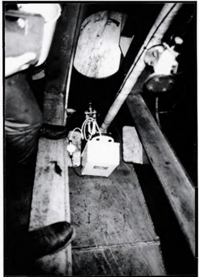
Plate 5: Aft sensor fixed directly to vent pipe – datum test valve positioned above the sensor
