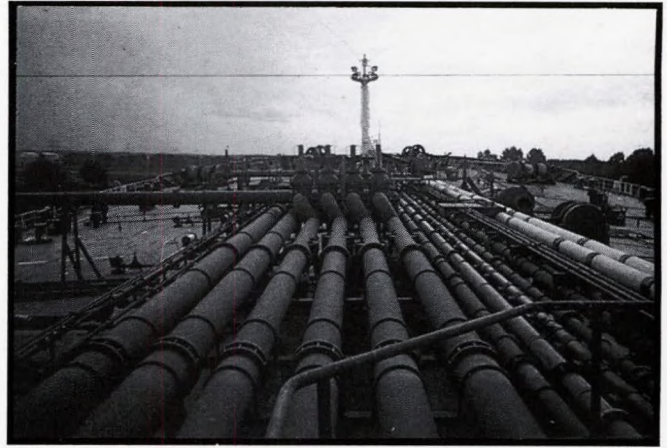
FIG. 3 Cargo lines on deck
