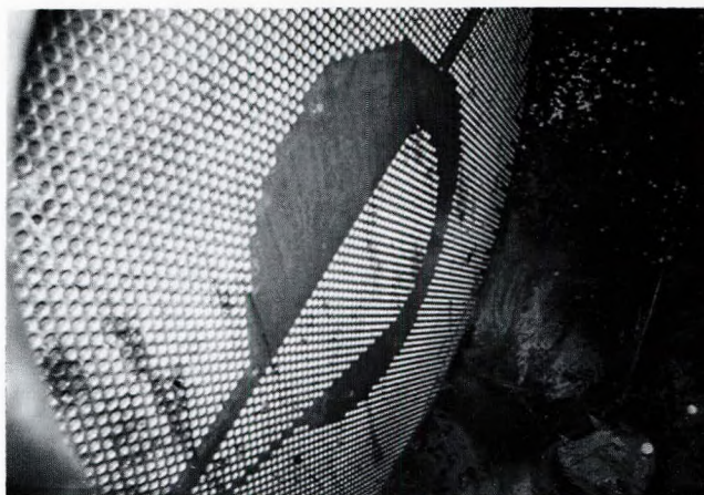
FIG. 10: Main-condenser inlet of the Limnea free of fouling
