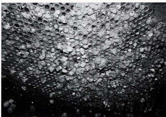
FIG. 11: Main-condenser inlet of the Latia heavily fouled following failure of the electrochlorination cells
