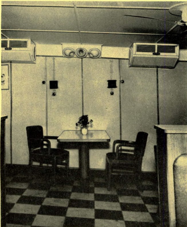
FIG. 15—Ceiling type cooling units can be served from central brine system or by direct expansion from semi-remote condensing unit
