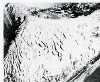
Fig 11 Dirty cargo tank
