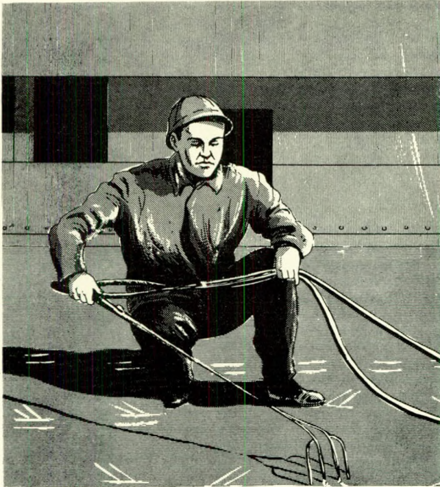
Heat is applied in spots with a welding torch; the flames are applied parallel to the beams, at 45 degrees, and finally at an inclination that gives the proper results.
