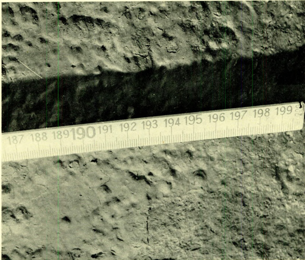
FIG. 6.—VIEW BETWEEN LOADED AND LIGHT WATERLINE: PAINT PARTLY DISAPPEARED (OCTOBER 1956). SCALE: FULL SIZE
