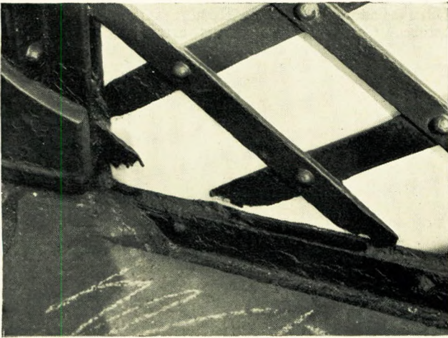
(a) PARAPET OF FOOTBRIDGE AT ST. JAMES'S PARK, LONDON The upturned members at the bottom have formed a trap for water, dirt, and rust, and the iron has corroded through there.
