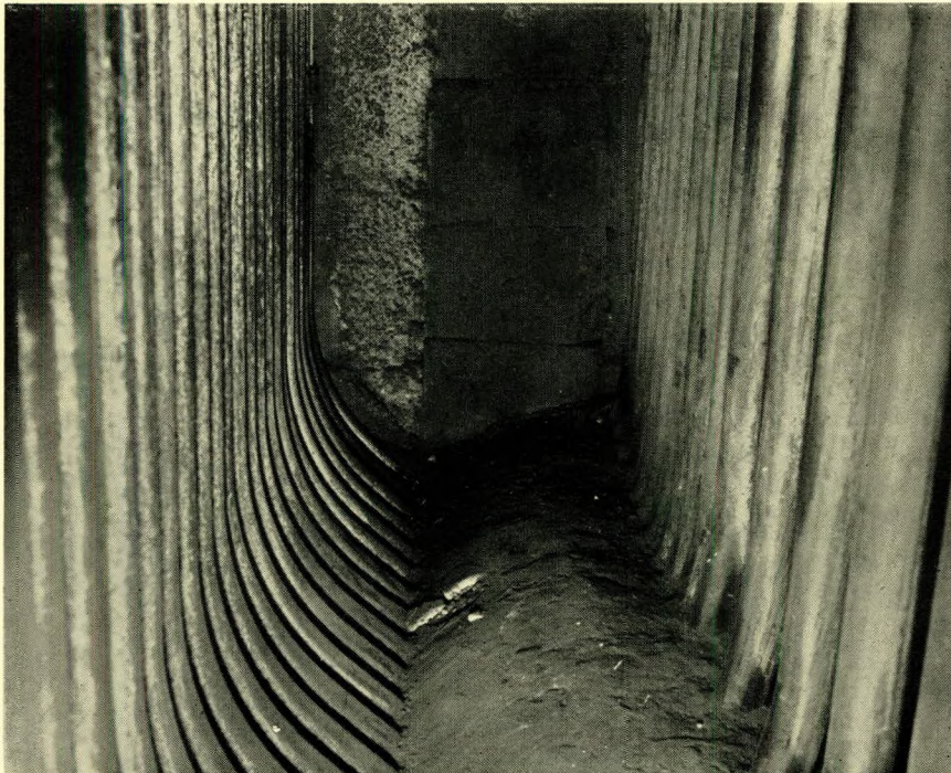
FIG. 6—Main boiler in s.s. Nestor: view between generating tube bank and starboard superheater support tubes (water drum)
