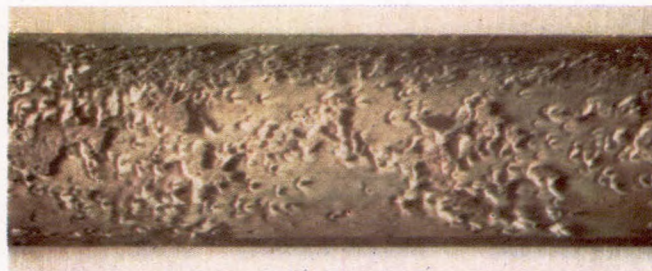
FIG. 7—70/30 brass generally attacked by corrosion erosion
