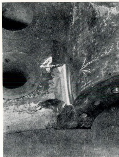
FIG. 29—Top half of h.p. cylinder: view of defect "D" chipped out for welding
