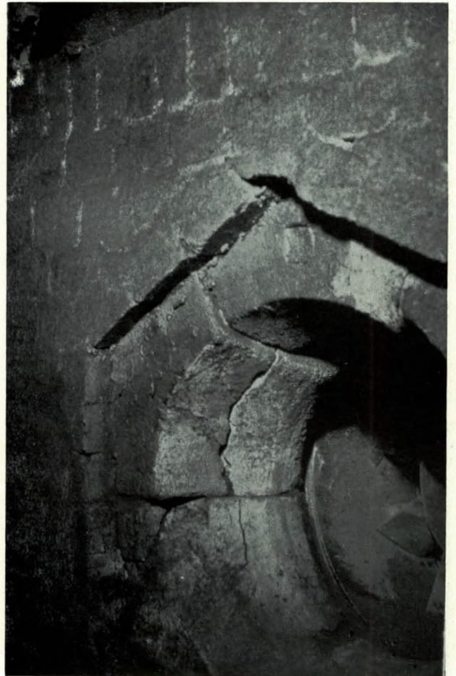
FIG. 16— Cracking of quarl blocks: header type boiler
