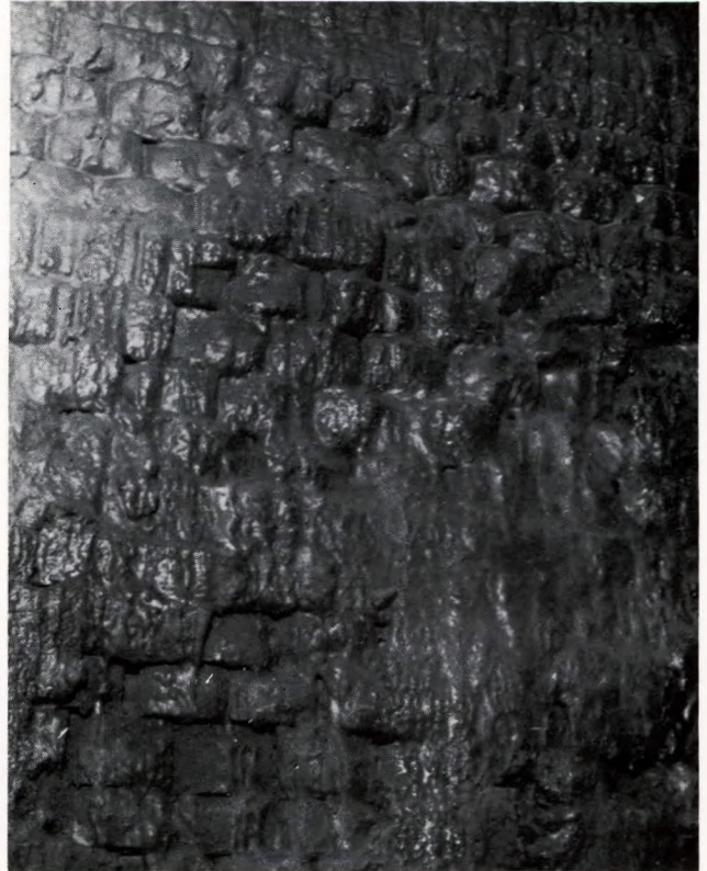
FIG. 10—Spalling damage to back wall of header type boiler
