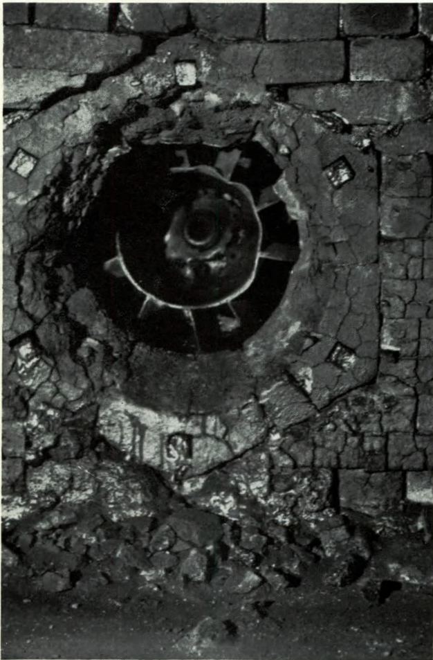
FIG. 15— Spalling damage to quarl blocks: header type boiler (six months' service)
