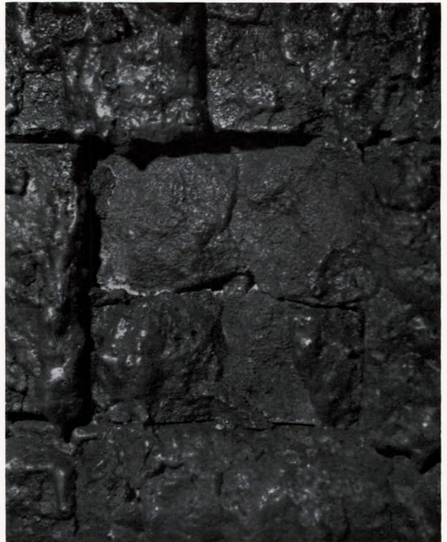
FIG. 12—Spalling damage to bolted blocks: end wall of end-fired Yarrow boiler
