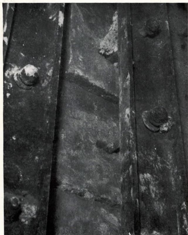
FIG. 24 (top left)—Damage due to failure of brick bolts: end wall of side-fired Yarrow boiler
