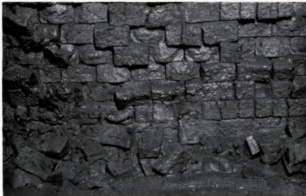
FIG. 11—Spalling damage to side wall of header type boiler I.Mar.E.1953]
