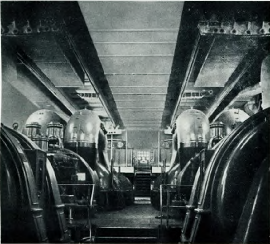
FIG. 3.—General view of turbine room.
