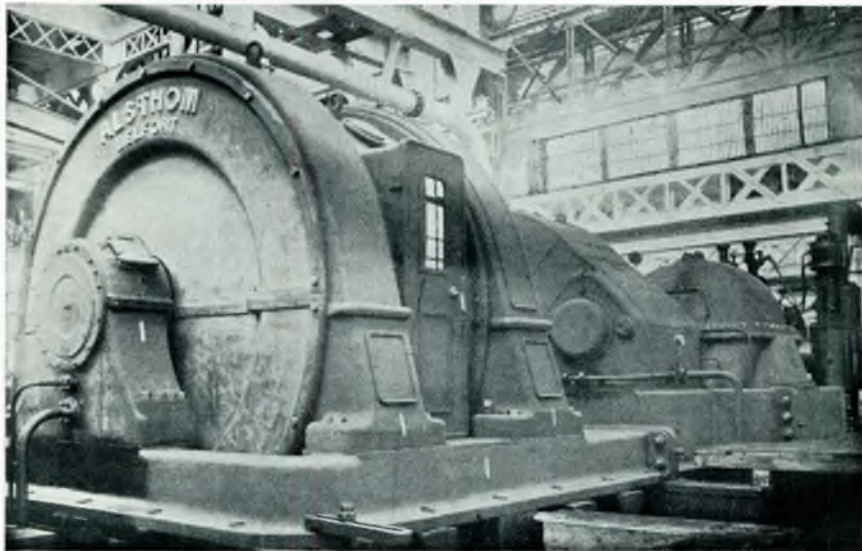
FIG. 10.—View of turbo-generator set—turbine end.
