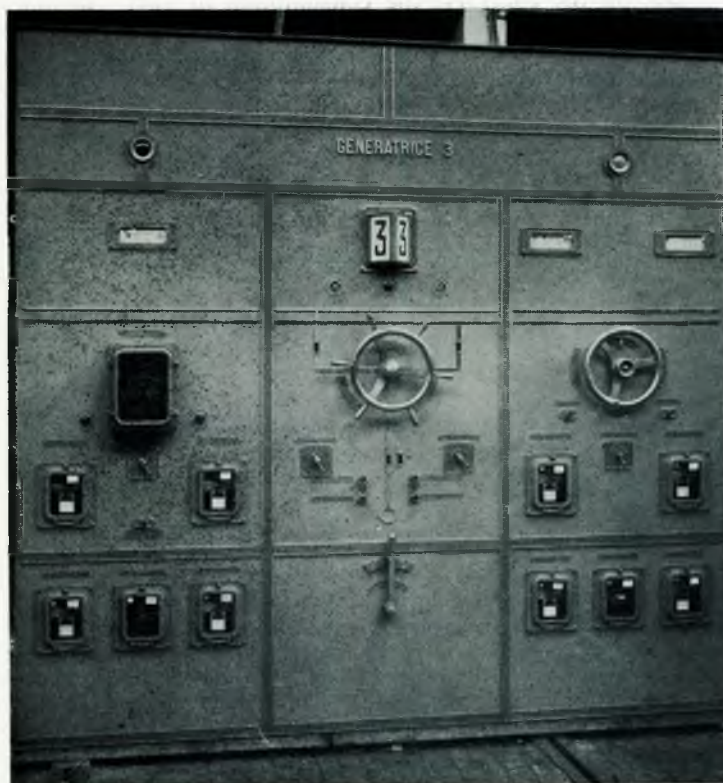
FIG. 12.—Detail view of main low-tension switchboard.
