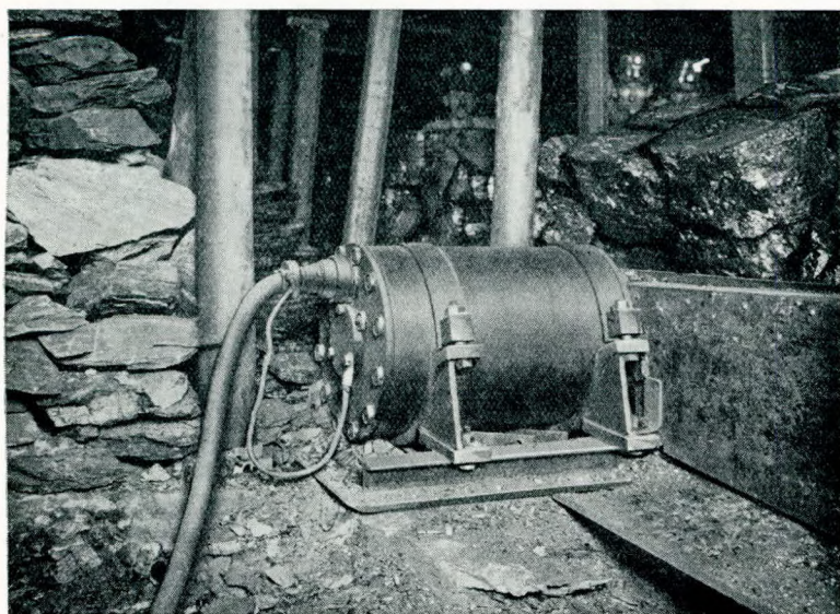
FIG. 7.—Flameproof squirrel cage induction motor driving chain conveyor in coal mine.
