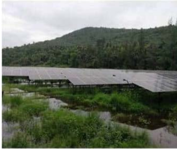
Figure 7: Solar Power Plants under Jawaharlal Nehru National Solar Mission
