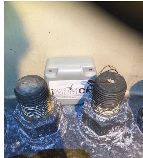
Fig.3: iWindCr system set-up in the MP-TP flanged connection location with the sensor attached to the M72 stud
