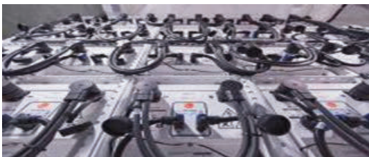
Figure 5. Battery modules storage system
