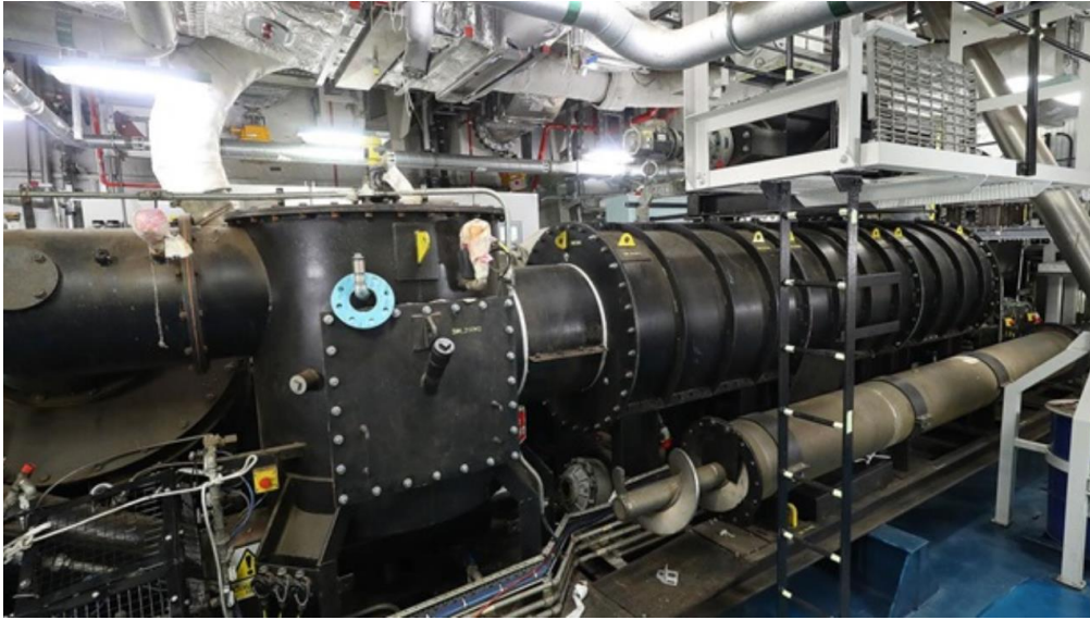
Figure 1: Pyrolysis plant, HMS Prince of Wales. Note the spare auger screw in foreground © Royal Navy 2019
