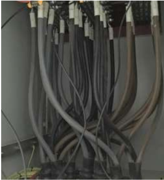
Figure 1–LV Switchboard Section (4000 A 4 MW)
