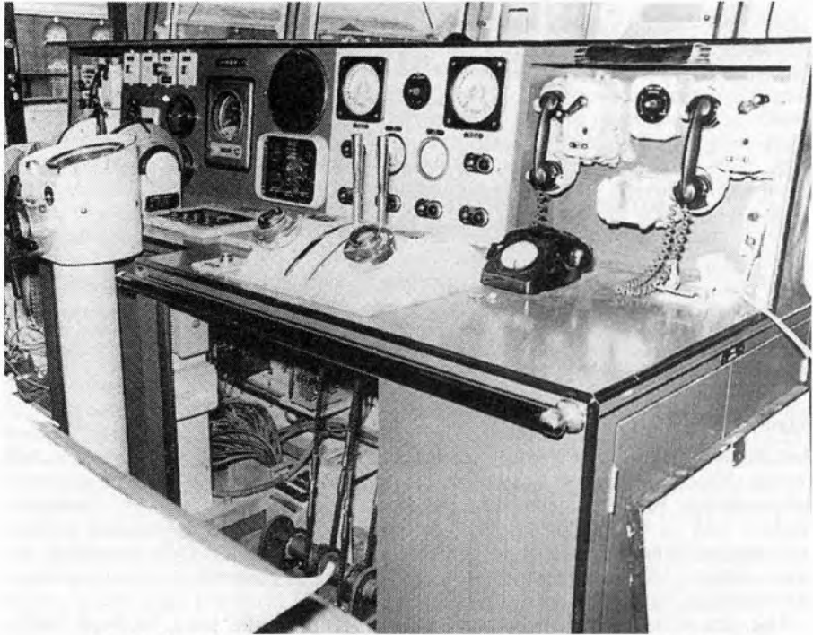
FIG. 2—PRESENT BRIDGE CONTROL CONSOLE, SHOWING MECHANICAL LINKAGE
