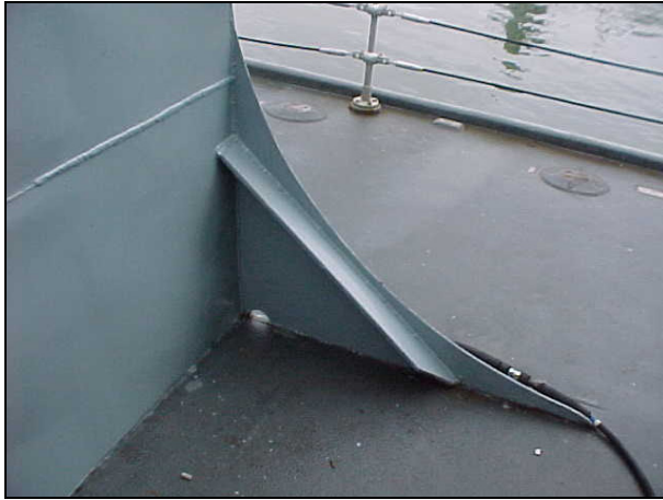
FIG.3 - T23 HANGAR BLOCK GUSSET PLATE
