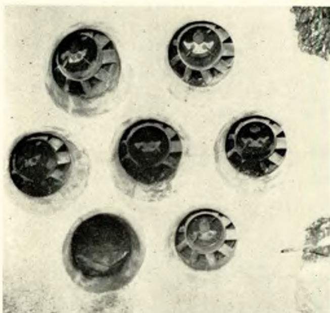
FIG. 5—Ship 2. Condition of front wall in December 1957
