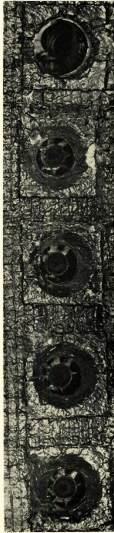
(b) Starboard boiler
