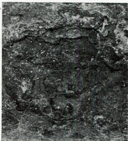
FIG. 1.—Scab pitting on the external surface of a fire tube in a Scotch boiler.
